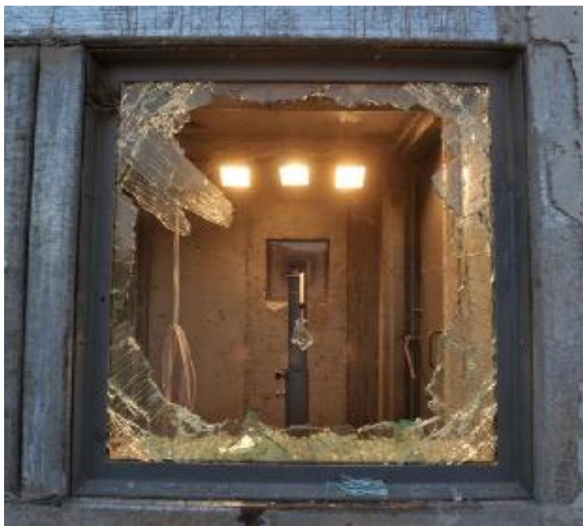
Figure 37 GFPM Target Broken Window Following Test 1
