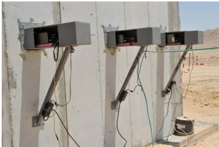
Figure 12 Camera instrumentation behind target
