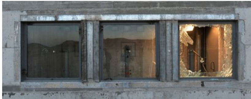
Figure 9 Glass pane fracture after first test
