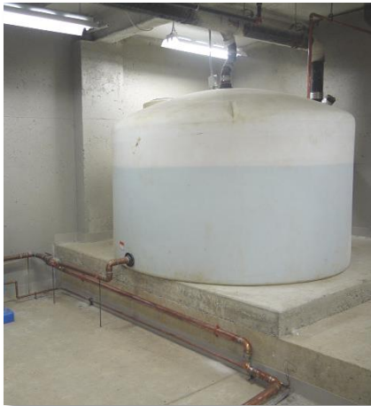
Rainwater Harvesting Tank
